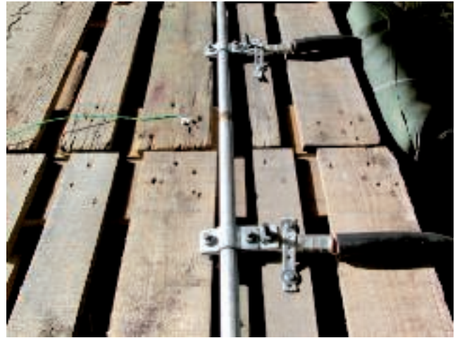
Short-circuit current test on earth rod
