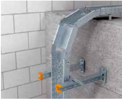
Mounting of falling adjustable vertical bend Mounting of the vertical adjustable bend, falling, to bridge height differences and changes from the horizontal to the vertical.
