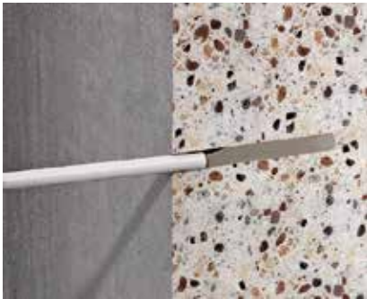
Application of the injection mortar Pressing of the injection mortar into the drill hole.
