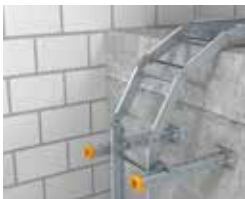
Welded cable ladder systems
