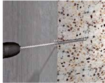
Cleaning with steel wire brush Mechanical cleaning of the drill hole with steel wire brush. The cleaning process with blowing and brushes must be carried out twice.
