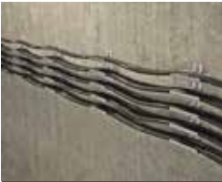
Cable support troughs
